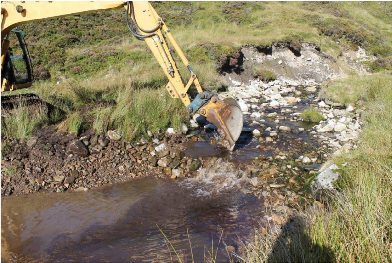
Figure 4.6. Wet excavation being conducted at a RoR hydropower scheme in a Scottish Highland catchment. Note that sediment removal is creating a headcut which could move upstream causing bed and bank erosion as it migrates and increasing sediment supply to the headpond.
