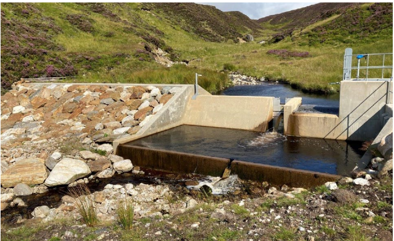
Figure 5.15. A Scottish Highlands RoR hydropower scheme. Photograph looking upstream.
