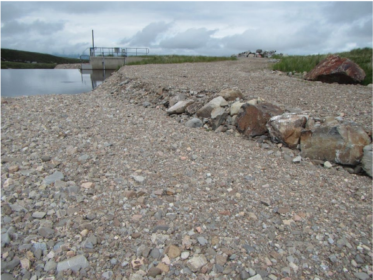
Figure 5.8. Pavement built on the right bank of the headpond of RoR Case study Two, using dredged material. Photograph looking downstream.
