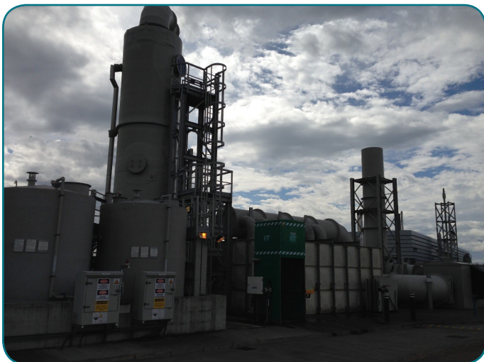
Figure 5: Chemical scrubber for air extracted from inlet works and primary tanks
