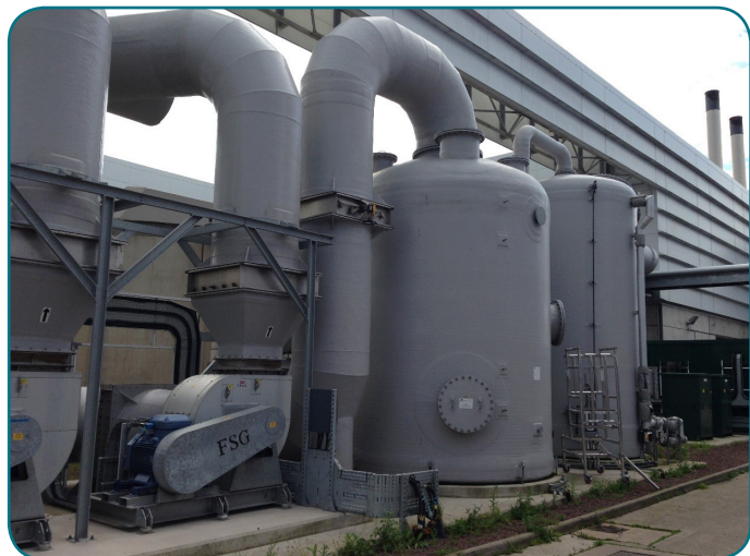
Figure 6: Activated carbon scrubber for air extracted from thermal hydrolysis sludge plant
