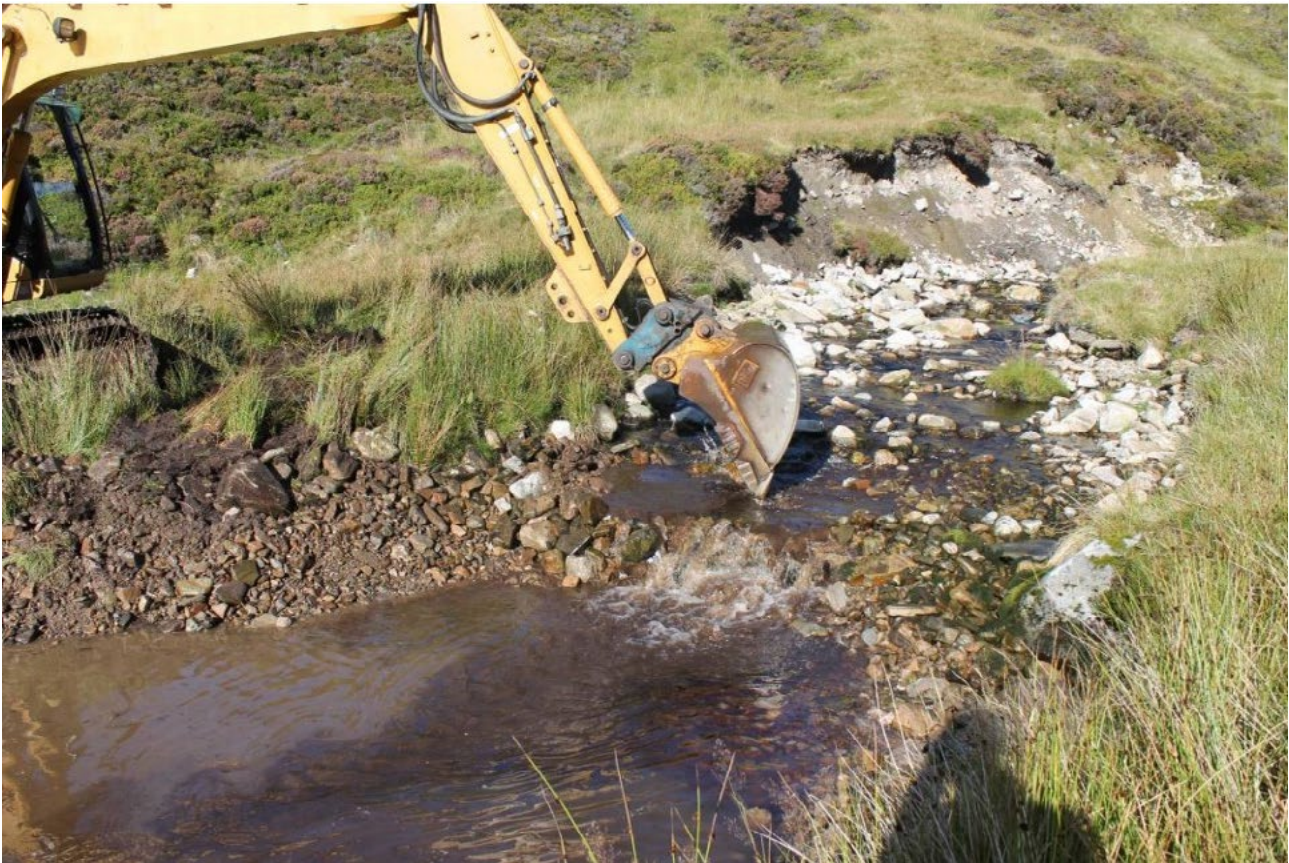
Figure 4.6. Wet excavation being conducted at a RoR hydropower scheme in a Scottish Highland catchment. Note that sediment removal is creating a headcut which could move upstream causing bed and bank erosion as it migrates and increasing sediment supply to the headpond.
